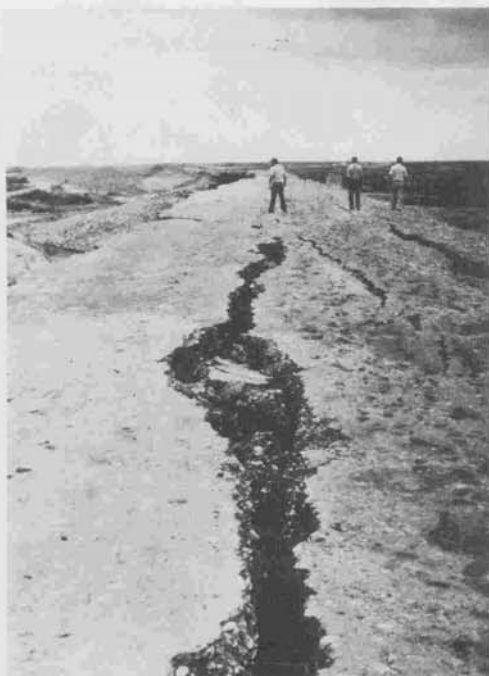
Tension cracks retrogressing behind slide scarp on remainder of crest and into upper part of downstream slope
